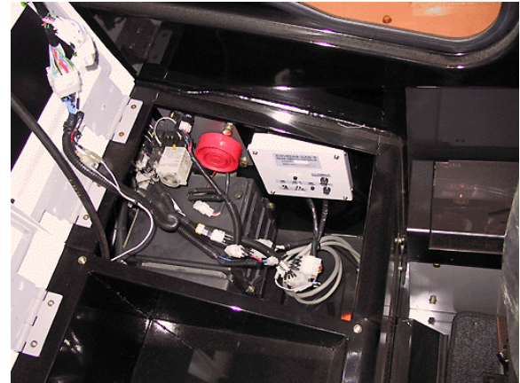
T4 / X91 / X94 Relay Location Behind Seat Under Panel
