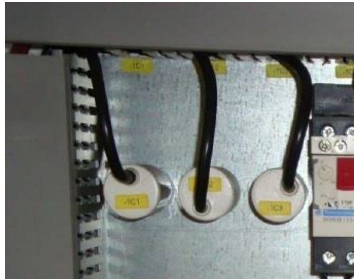
Capacitors in B Panel
